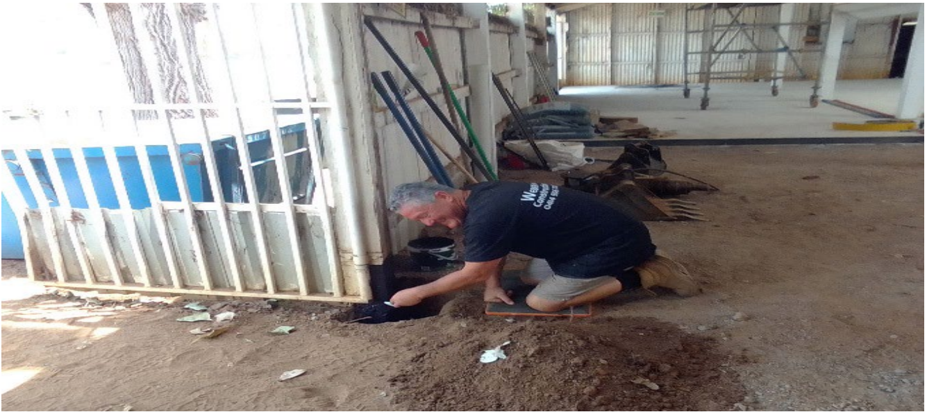
Tony completing subsurface waterproofing of the 48 th Post. “The Last Post” Yes a bugler was playing!!
